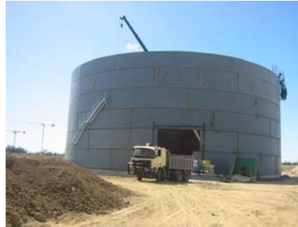
42.0m dia x 20.0m high Cone Roof API Tank – BP, Mackay
