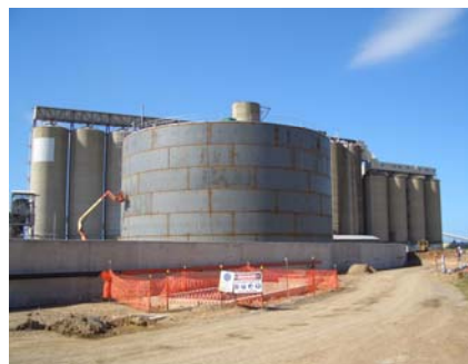
34.3m dia x 18.0m high Tank with Self Supporting Truss Roof Caltex, Gladstone
