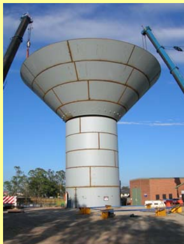
Kellyville – Cone Lift 130 tonne x 23m dia
