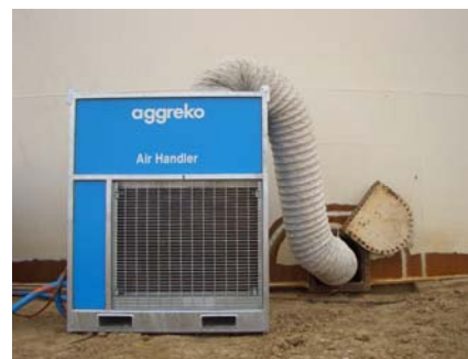
One of a number of refrigeration units used to cool air inside Tank 3000
