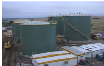
Port Campbell Tank Farm
