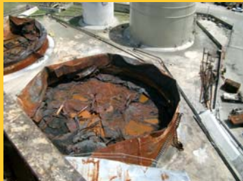
Fire Damaged Tank in Guam
